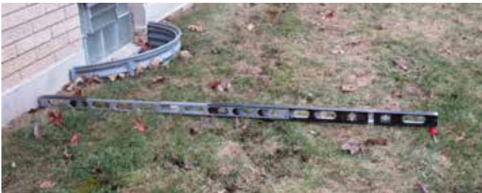
Figure 5: Poor Surface Drainage
