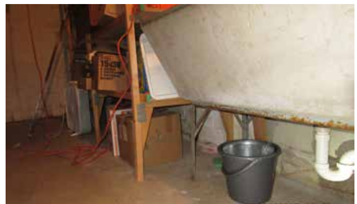
Figure 3: Basement Leak at Lower Block
