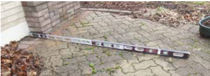
Figure 6: Poor Patio Drainage
