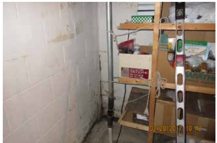
Figure 2: Basement Leak High on Wall
